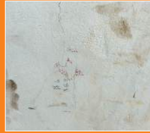
3. MARKING OF SAMPLE CRACKS
